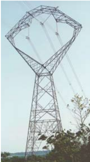
Internal compact delta, 500 kV
