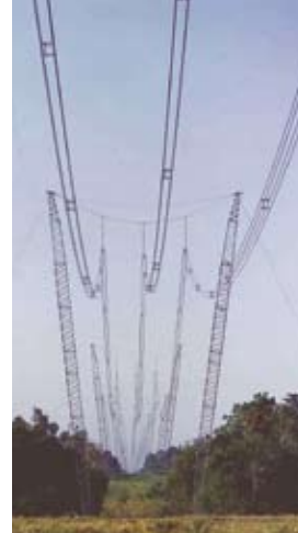
Crossrope suspension, 500 kV
